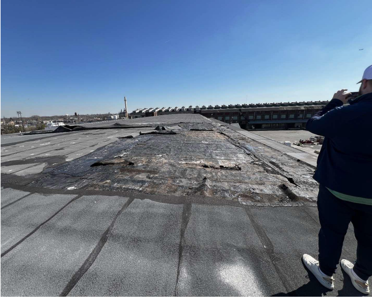
Y-2 Building – Damaged Area - Looking East
