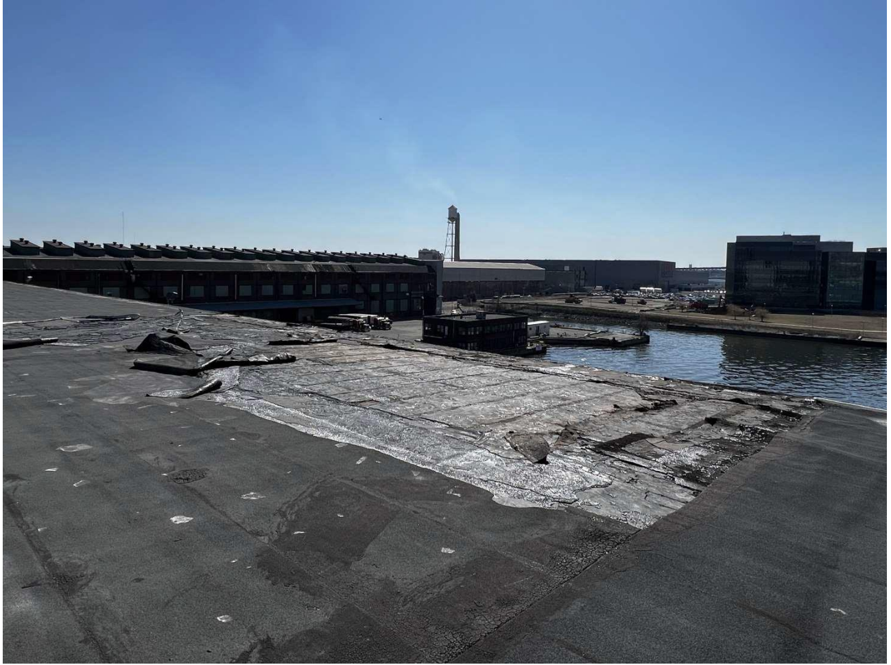
Y-2 Building – Damaged Area - Looking Southeast
