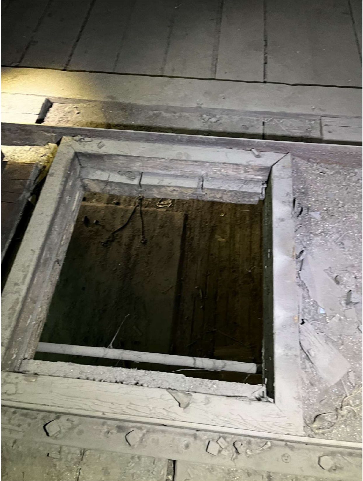
Photo No. 2 - Typical Ceiling Hatch - Looking Down from Attic Space above West Gallery
