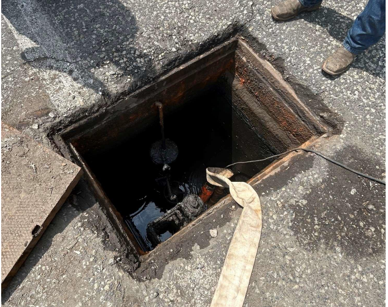
Flushing Station with Air Relief Valve
