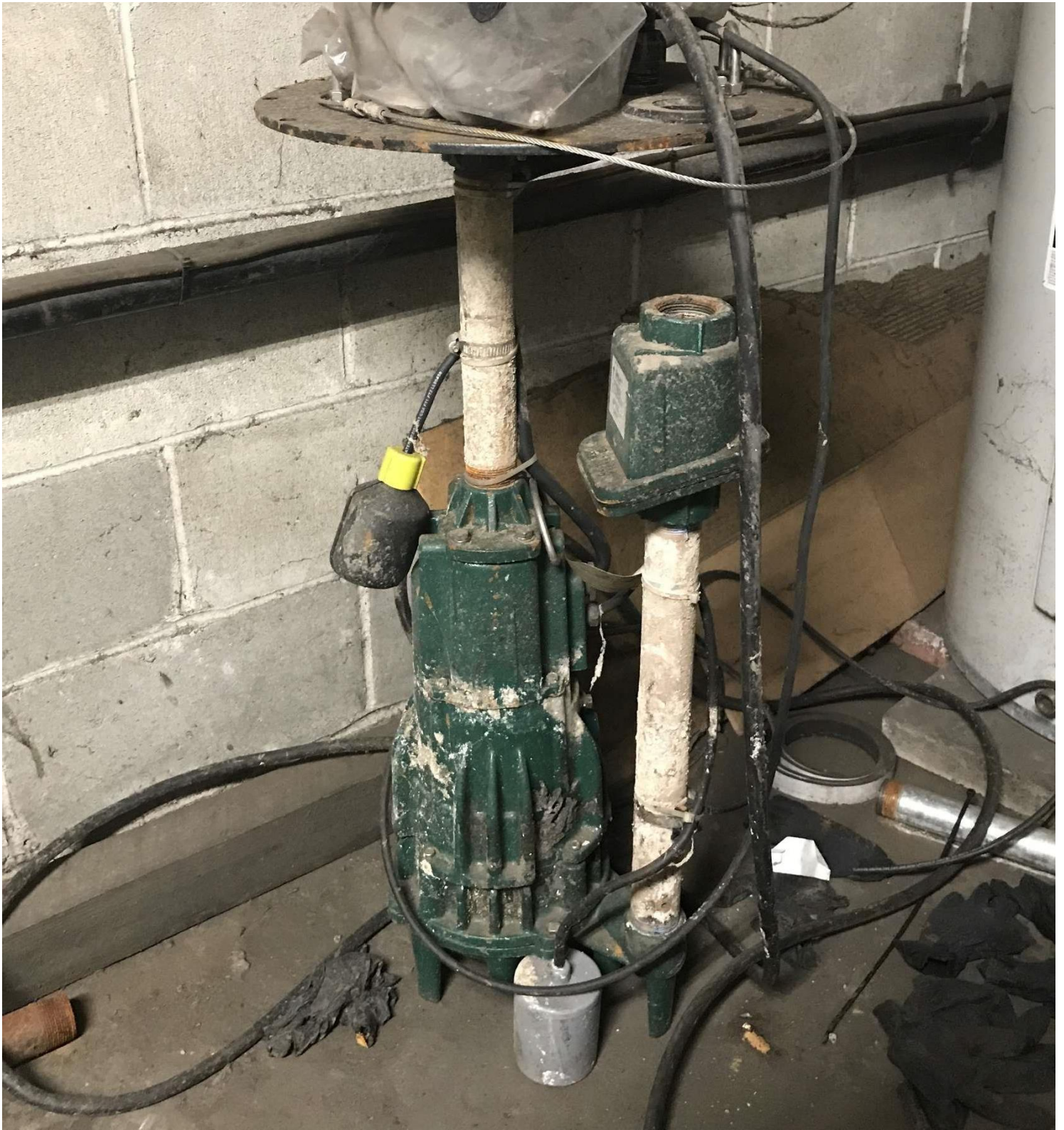
Existing Grinder Pump
