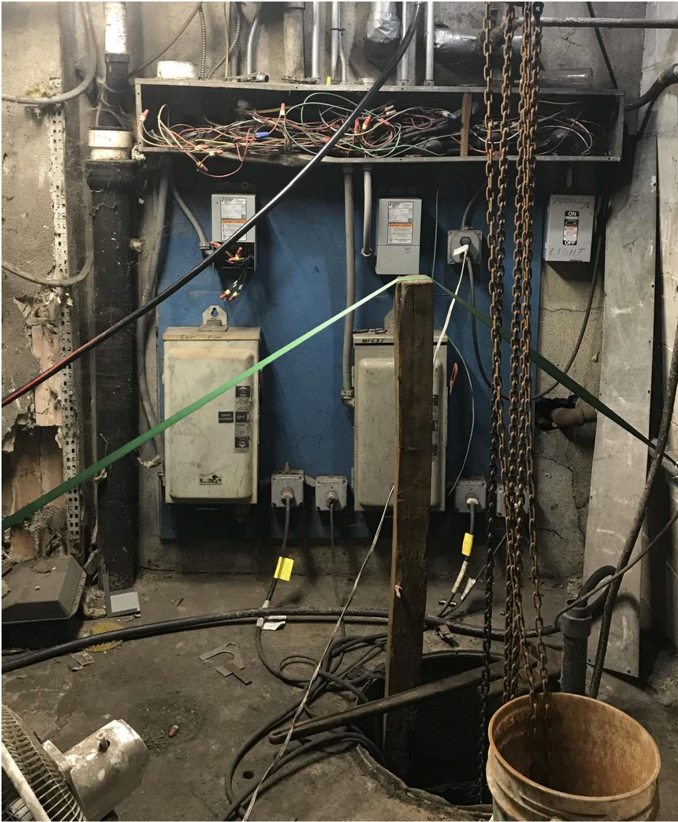
Existing Controls Panel
