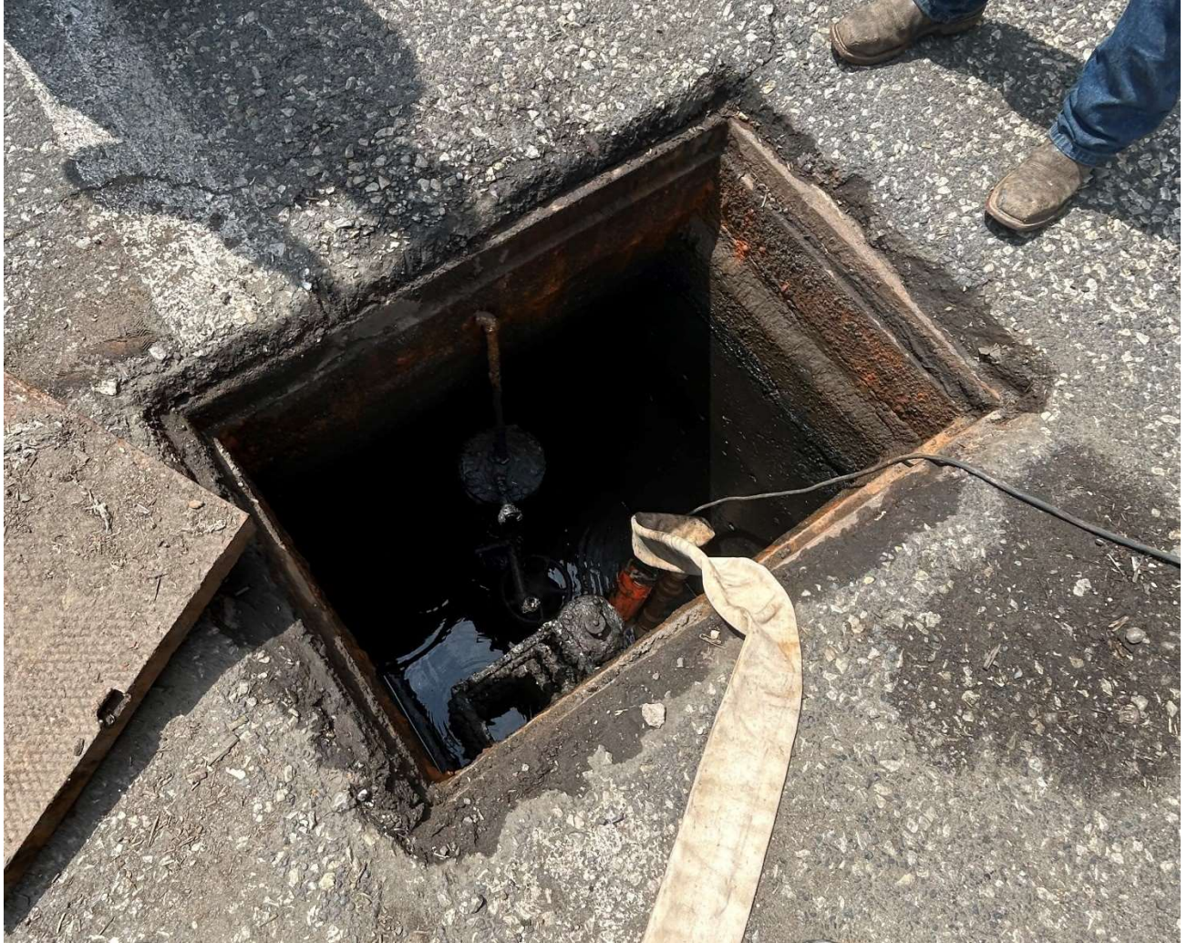
Flushing Station with Air Relief Valve
