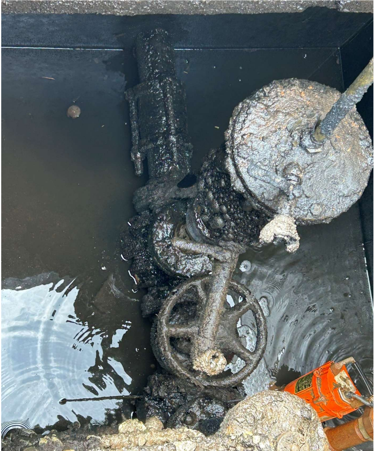
Flushing Station with Air Relief Valve
