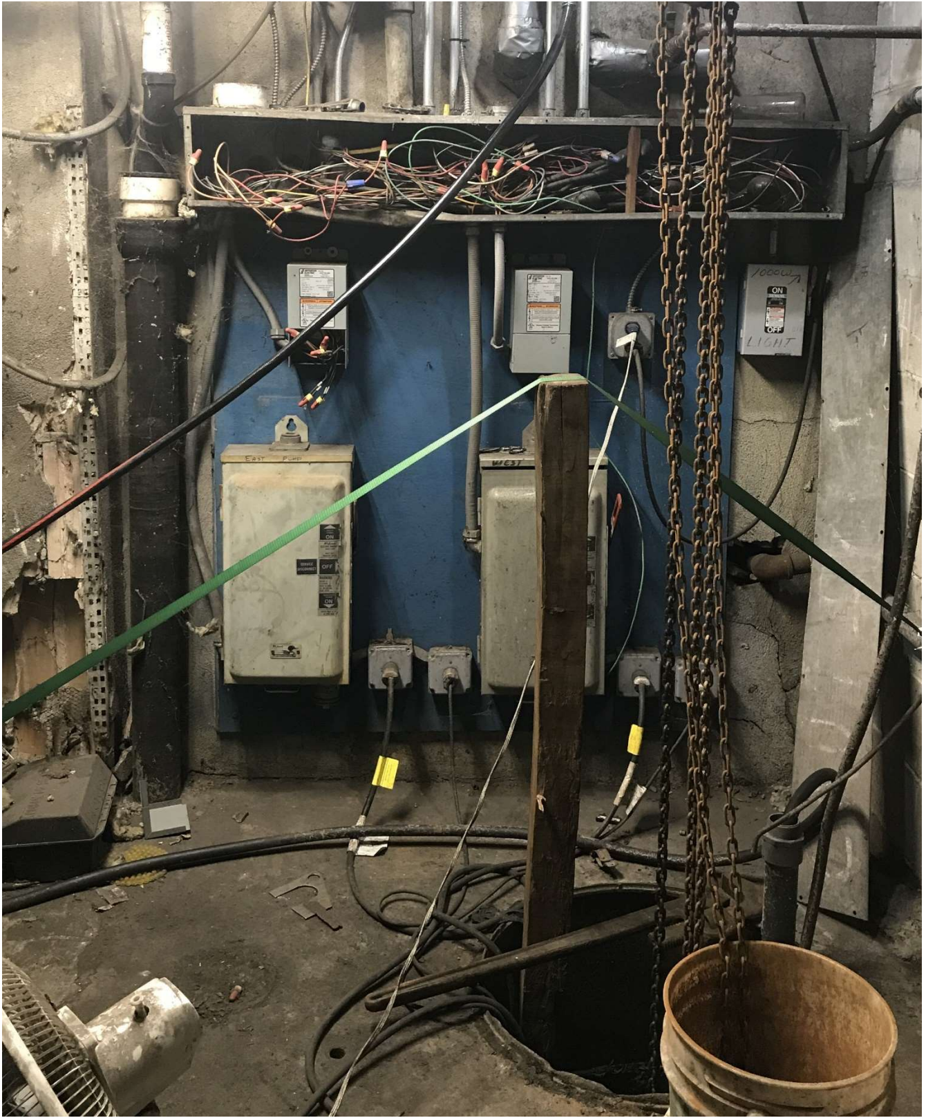
Existing Electrical Panel
