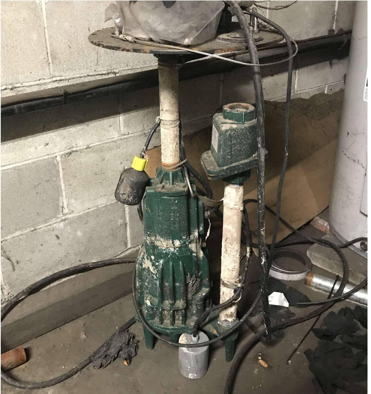
Existing Grinder Pump
