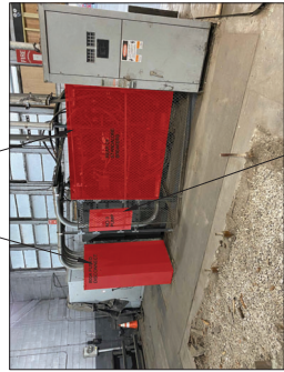
NO 3 PUMP HOUSE
