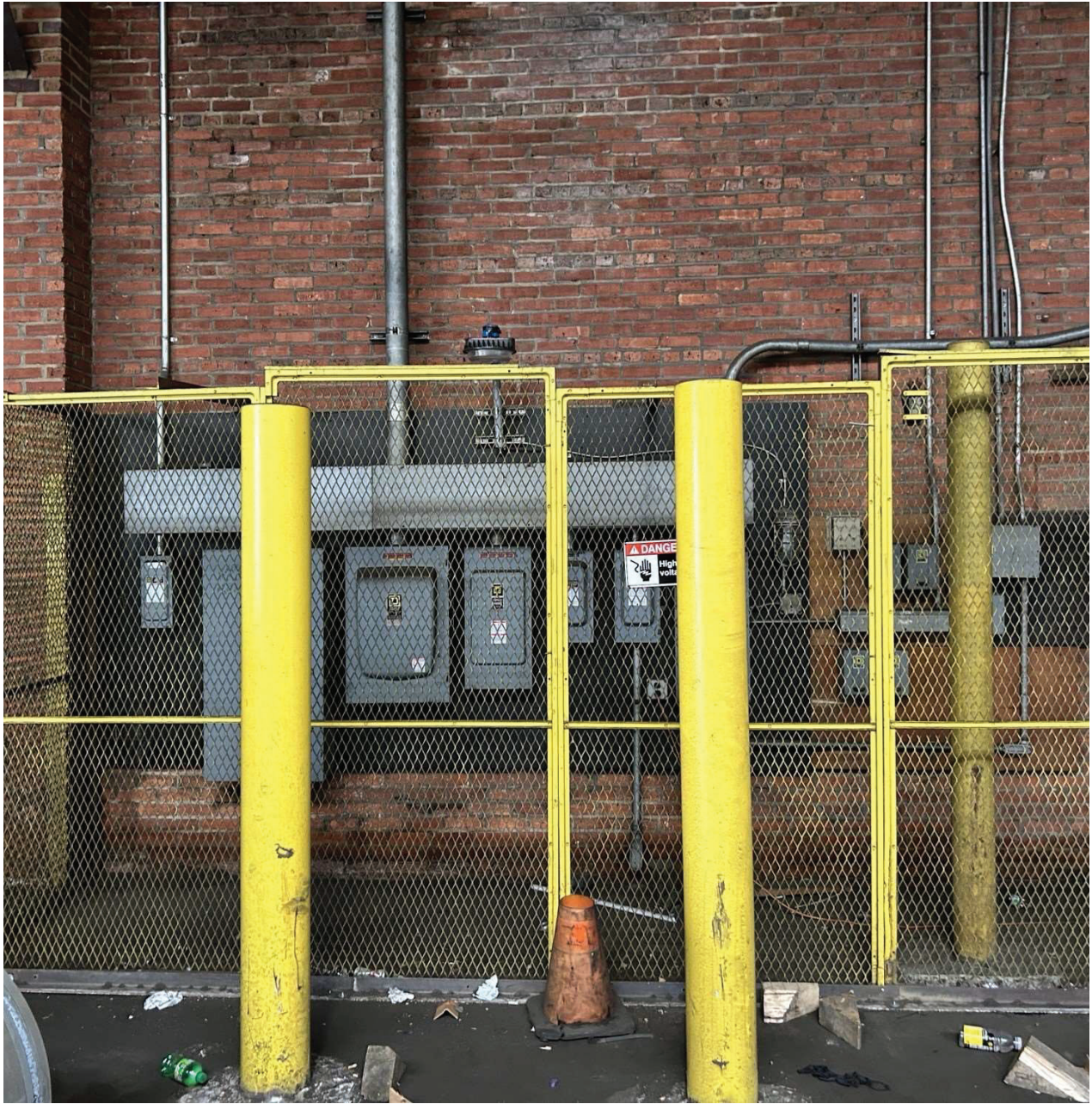
3. Existing Upstream Disconnect Panel is located here.
