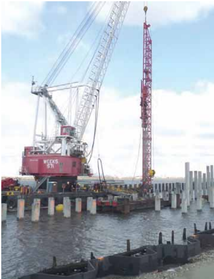
Both photos: Pilings being driven for the wharf at the SJPC's new omniport in Paulsboro.
