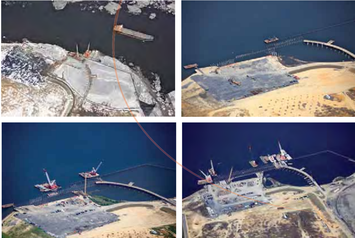
Progress at Paulsboro: These aerial photographs show the progress on wharf construction during 2015, clockwise from top left, are shown January through April, July and November.
